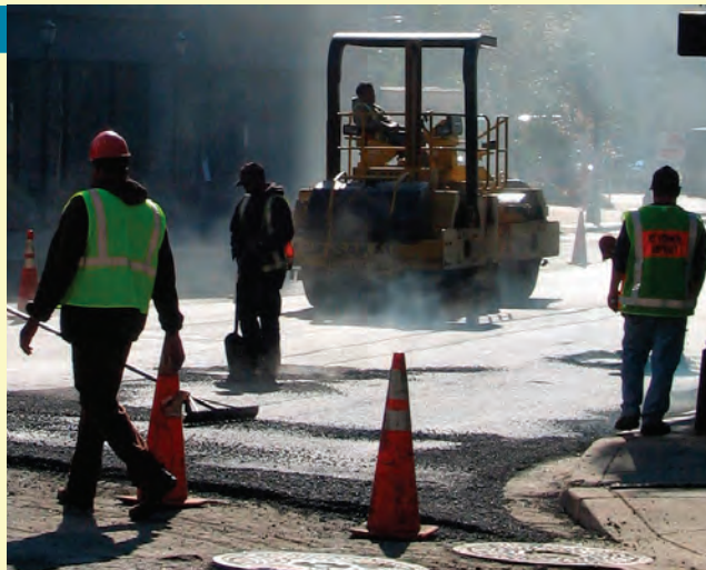
When highway engineers design and build highways, they must know the grade, or slope of the road.
