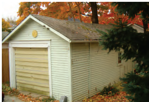
The roof of a garage gains strength and stability from its triangular form. By supporting a roof with triangular trusses, the roof is made even stronger.
