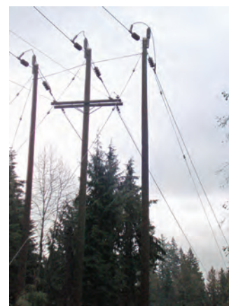
Guy wires add stability to poles carrying electrical lines.
