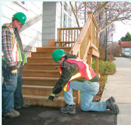
Determining the angle of elevation of a staircase is an important step in its design and construction.
