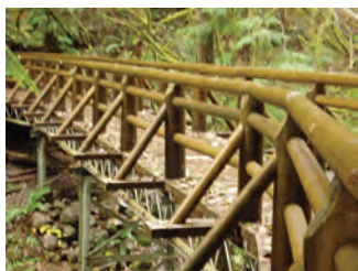
The railings and supports of this bridge are reinforced with right triangles.
