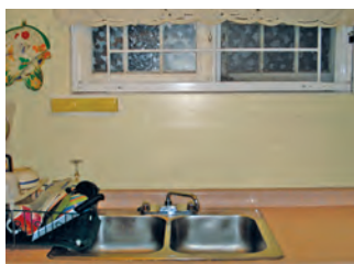
New kitchen countertop can be cut to the correct size with a jigsaw. If the countertop contains a sink, silicone sealant must be applied where the countertop and sink meet.
