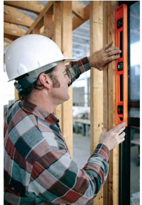
A glazier uses a level to ensure that the window will be straight.
