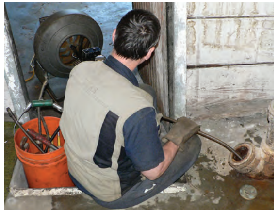
One of a plumber's tasks is to remove roots from drains with a snake.
